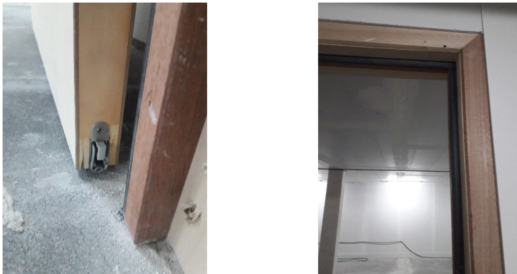
Figure 7: Smoke control door (drop sill – left; rubber seal – right)
