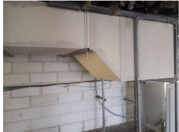
Transition rectangular duct to fan
